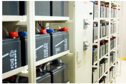
UPS battery racks
