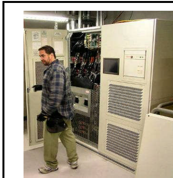
500 kVA UPS w/o batteries
